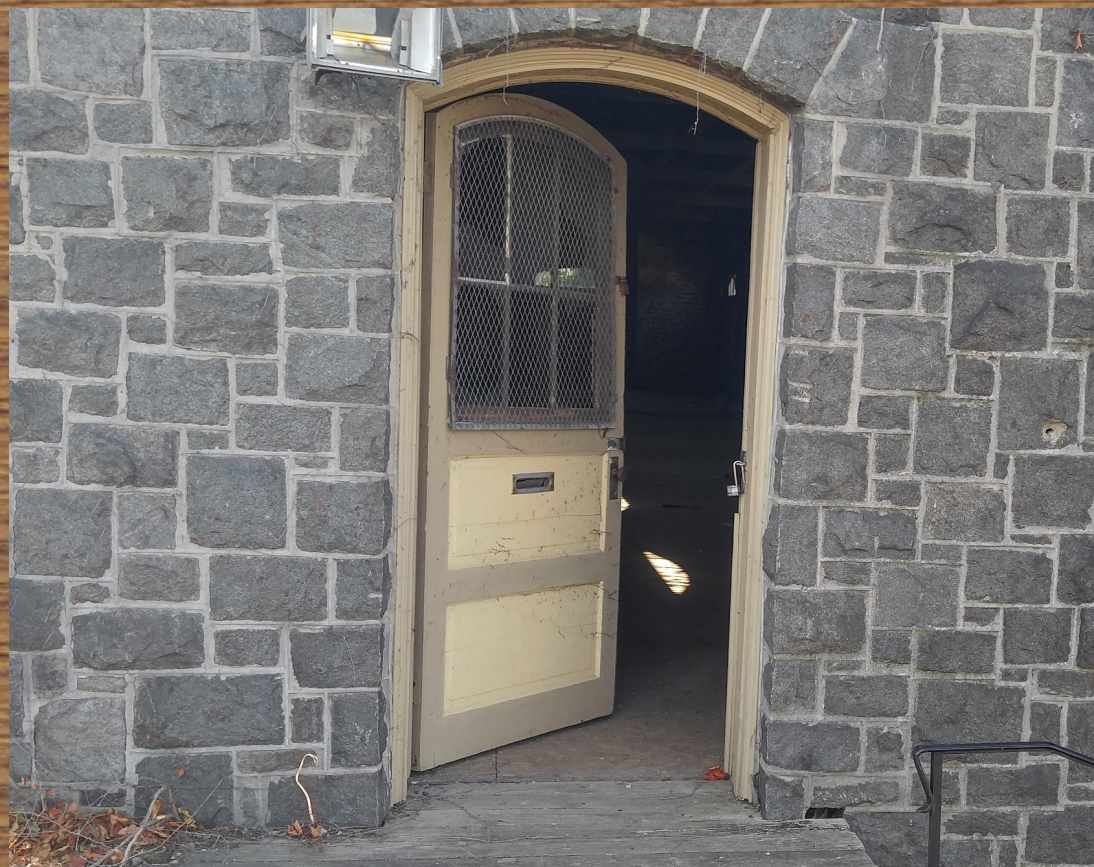
Front door: Missing glass, misaligned
