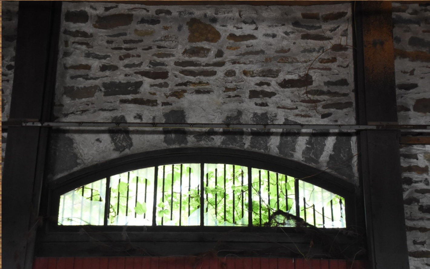
Transom windows broken, frame in poor condition
