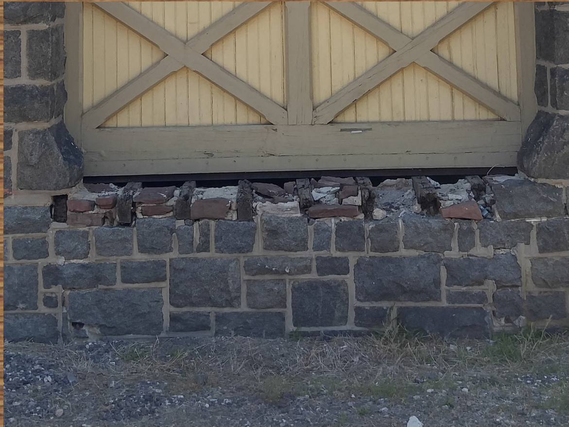
Exposed joists at freight doors
