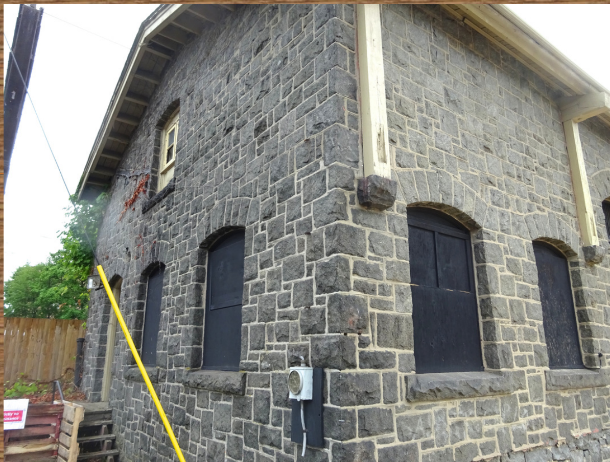
Windows boarded up, in poor shape
